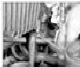
8.16f Uncover the fuel exhaust intake control secured using bolts
