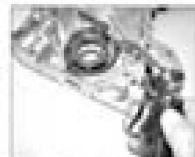
10.9a Thoroughly lubricate the pump internal components with clean engine oil, then add the pump cover.
