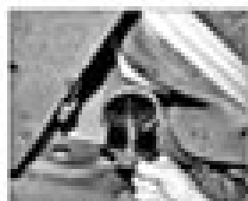
10.4a Use a screw to pull the old filter from the housing.
