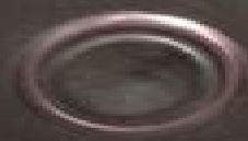
push button for indication of pressure before oil separator
